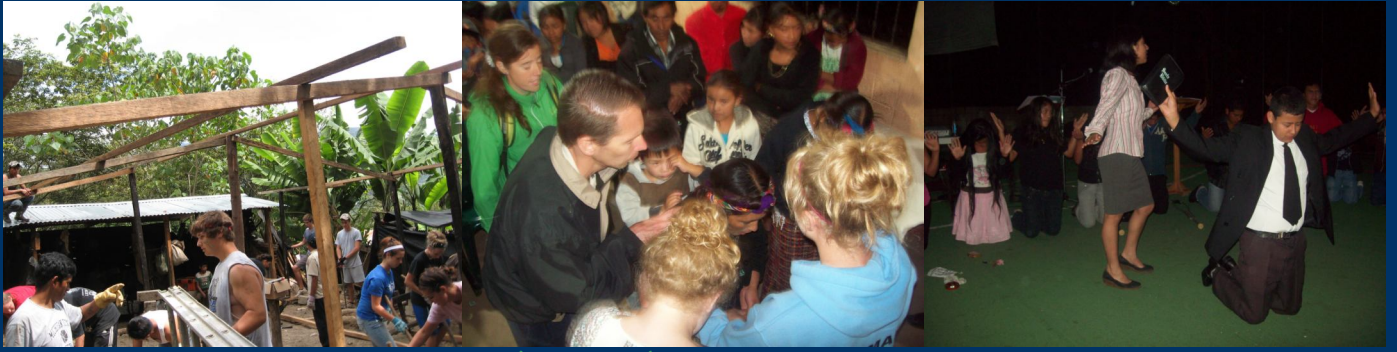
Early July: Resurrection Life Church (Michigan) came for a few days thanks to ASELMI ministries (Bible Institute ministry that we are part of). Pictured here: putting a new roof on a needy family's home, prayer at altar call during a youth rally, a local church performs a drama skit during another rally.
